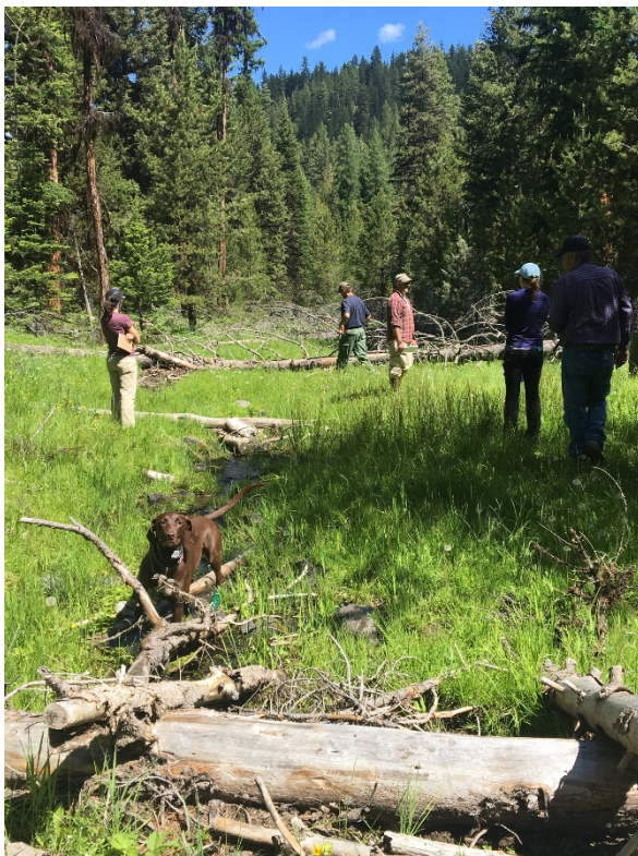
Upper reaches of Camp Creek looking downstream at trees and debris placed across the creek.
