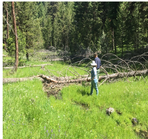
Another view looking downstream with trees cut to fall across the stream to spread high water and increase soil deposition.
